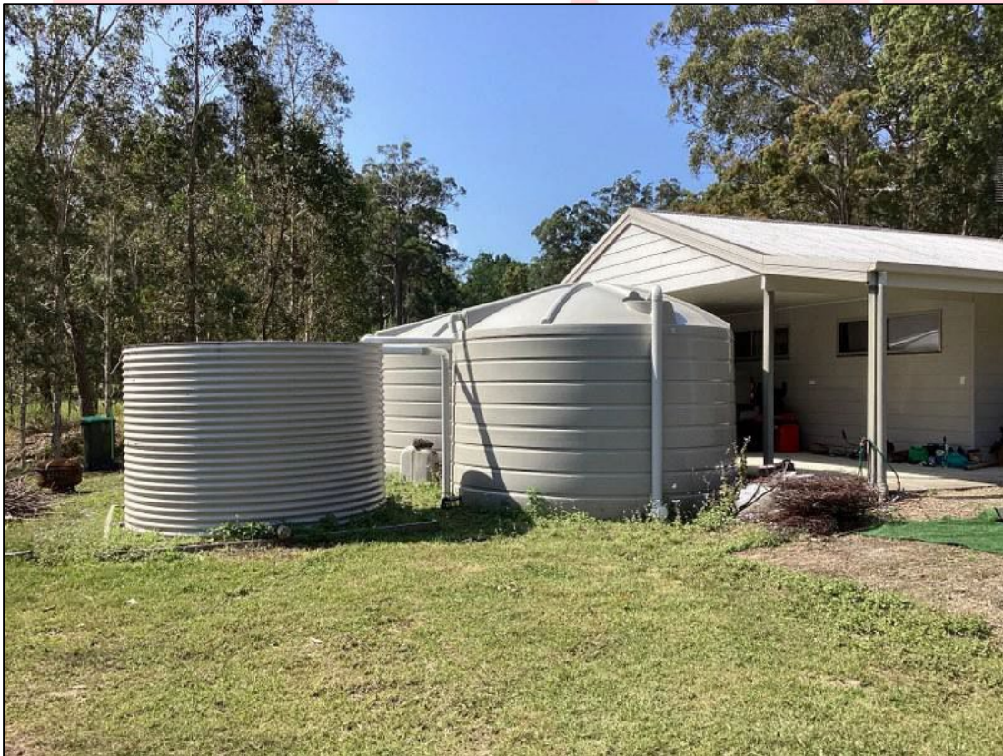
Plate 4 (P4) Compliant Static water supply to existing dwelling on proposed lot 1
