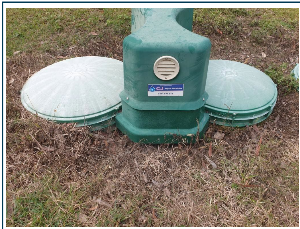
Photograph 1 – View of the existing AWTS located to the north of the existing dwelling.
